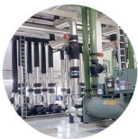
HV AC Air conditioning
